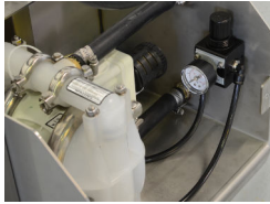
Pressure regulator and double membrane pump
