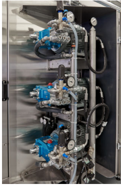
High-pressure pump system
