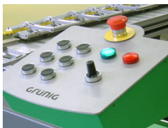
Control panel A1
